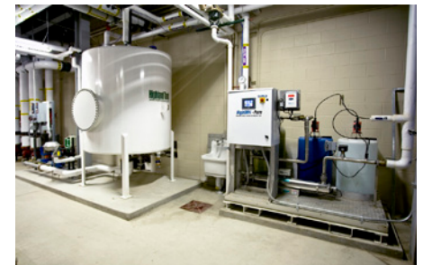
Rainwater Harvesting Systems
